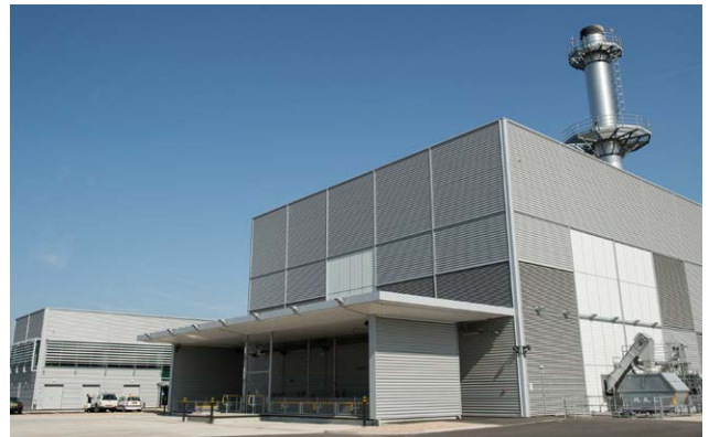
Biomass boiler at Heathrow Airport
