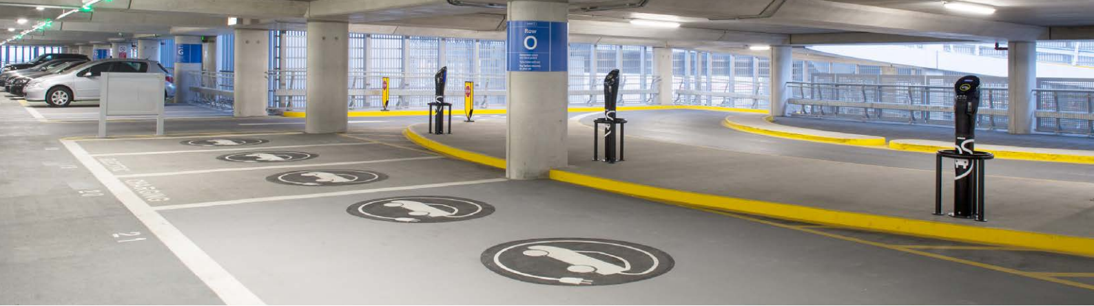
EV charging facilities at Heathrow Airport's passenger car parks
