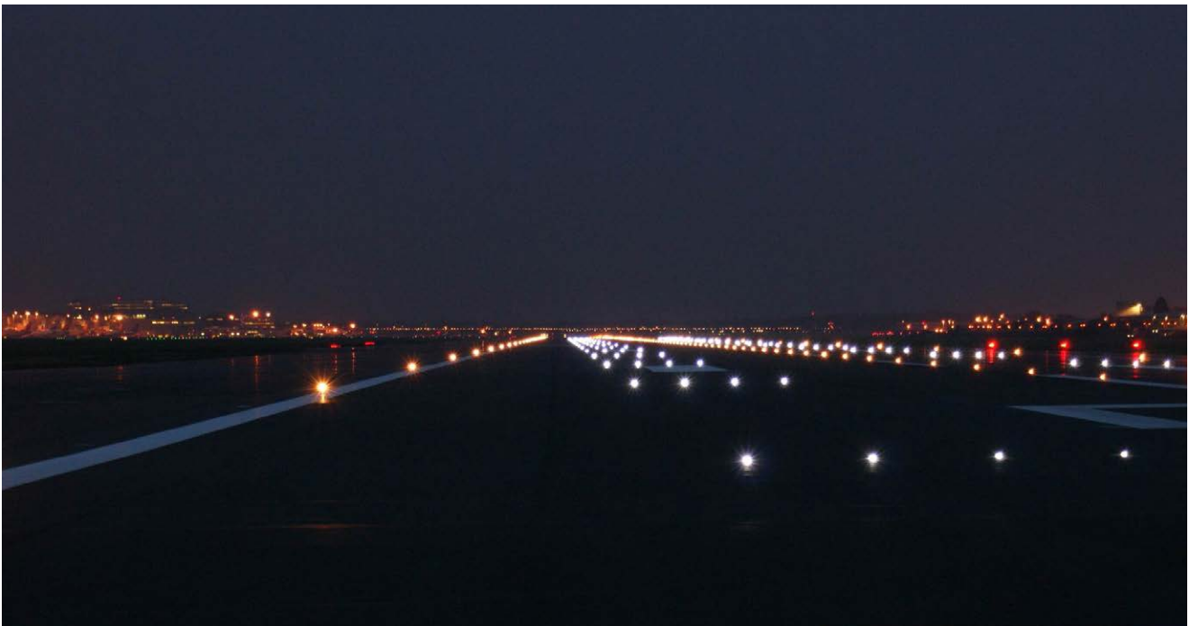
LED lights in operation at London Gatwick Airport
