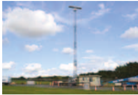
LightWave Radar installed at Glasgow Prestwick Airport for pre-certification testing
