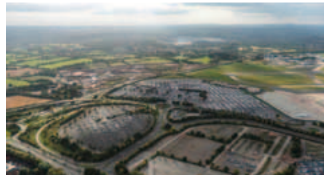
Birmingham Airport’s 405m operational runway extension is being constructed by the VolkerFitzpatrick Colas Joint Venture.
